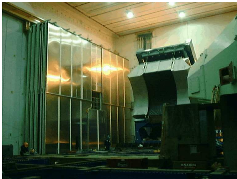
Figure 2.22: The south PHENIX Muon Identifier before installation of the shield wall.
